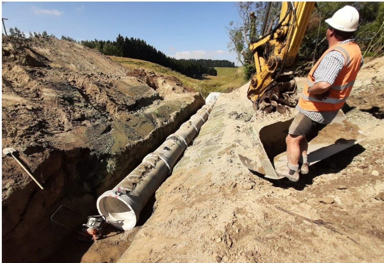
Figure 5 Airedale Road sinkhole
