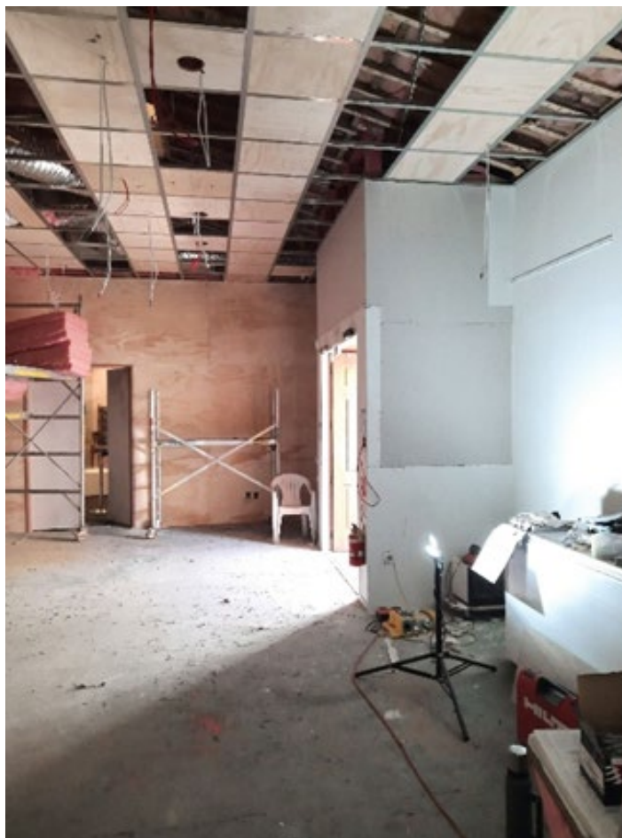
The archive enquiry area as work on the new ceiling and wall linings is completed.
